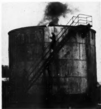
APPLYING TORCH. —Workman at Socony-Vacuum's Olean, N. Y., refinery, applies torch to 100,000-gal. tank of kerosine.
